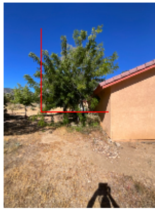
Vegetation, touching rear side of structure
