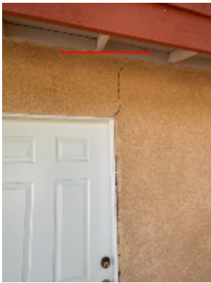
Hairline crack on garage. on garage exit door exterior
