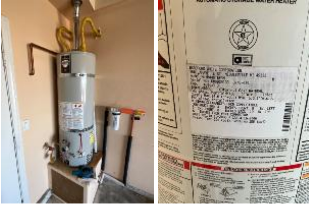
Direct view of water heater Water heater service tag
