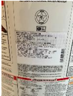
Water heater service tag
