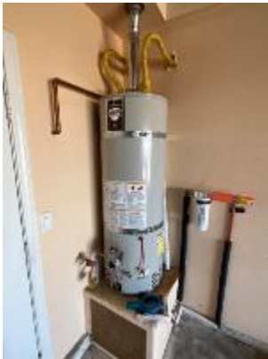
Direct view of water heater
