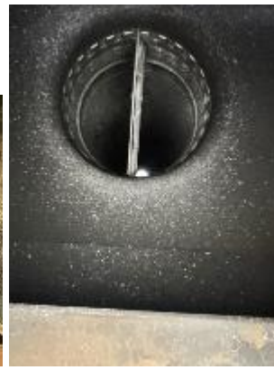
Fireplace damper door in open position
