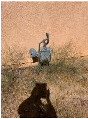
Direct view of gas meter
